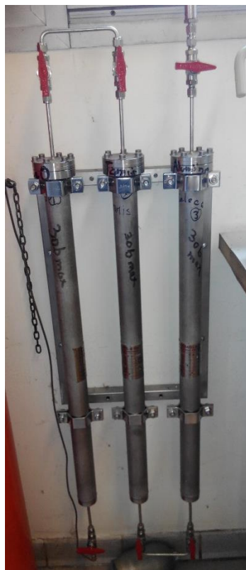
Figure 17 - Propylene purification columns.
